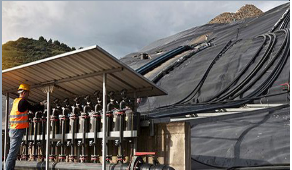
Biogas and biomass energy plant (Photo courtesy of Parker.com)
